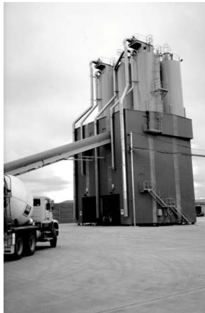
Measurement in 14 m silos containing cement, fly-ash and other ingredients for concrete manufacturing
